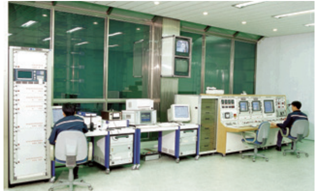
Control Room of Ultra-High Voltage Test Laboratory
